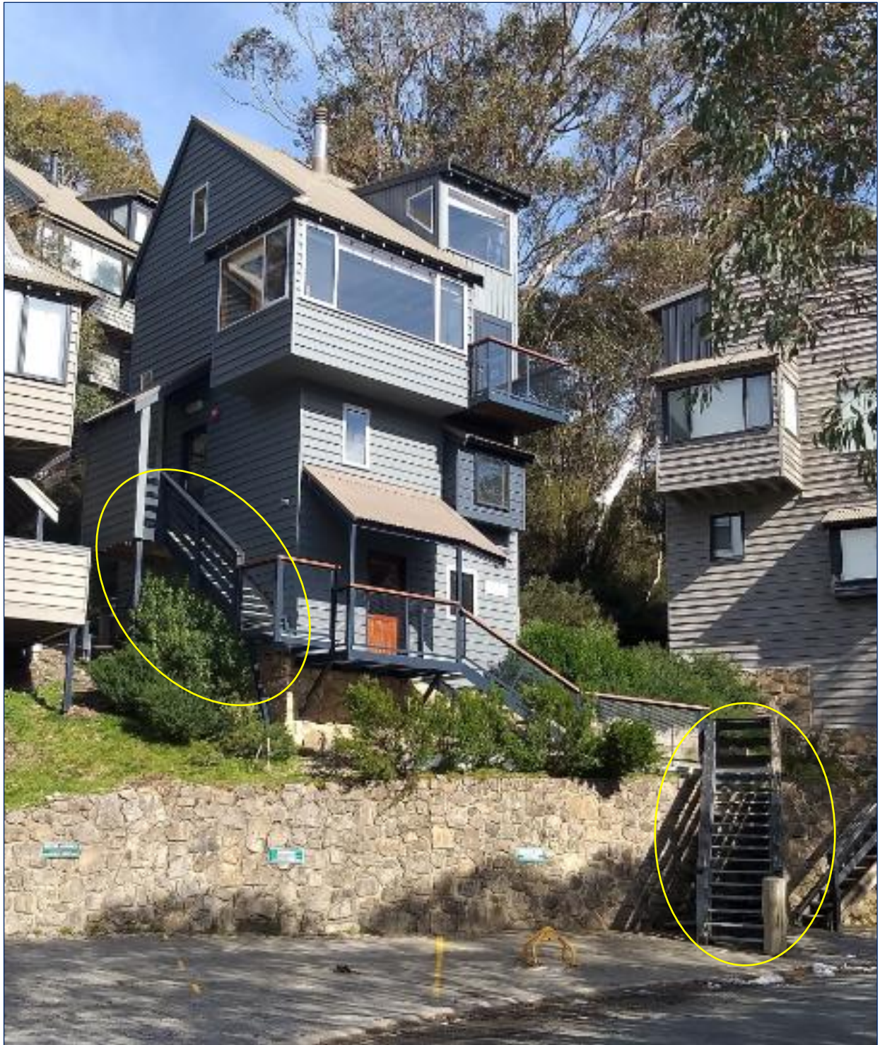
Figure 2 | Chimneys Ridge viewed from Diggings Terrace, illustrating external access staircase to be partly replaced (Source: Department inspection)
