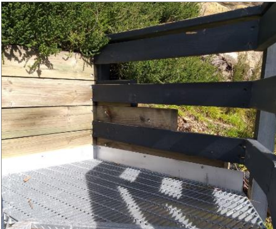
Figure 5 | Existing sleepers and stringers / handrail to be replaced (Source: Applicant's documentation)
