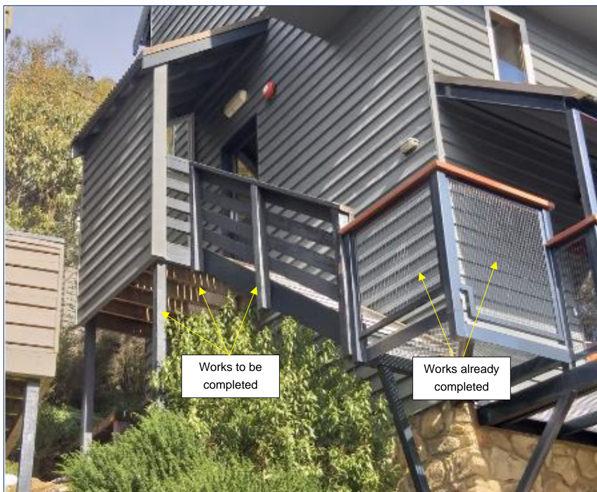
Figure 3 | Existing landing, stringers and handrail to be replaced as per below works already undertaken (Source: Department inspection)
